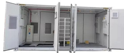
1075KW HH ESS
