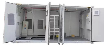
1075KW HH ESS
